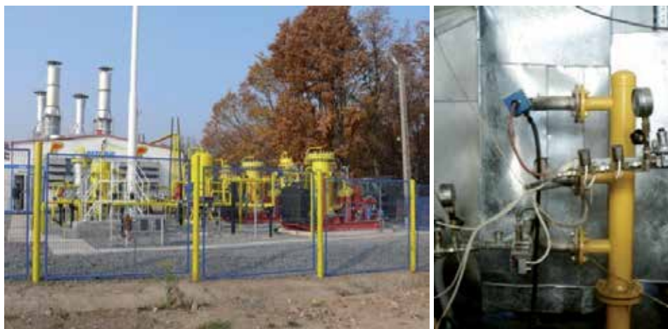
Figure 2. Cogenerative plant 2xST 18 – Suplacu de Barcau (left) and afterburning installation (right) [14, 15]
