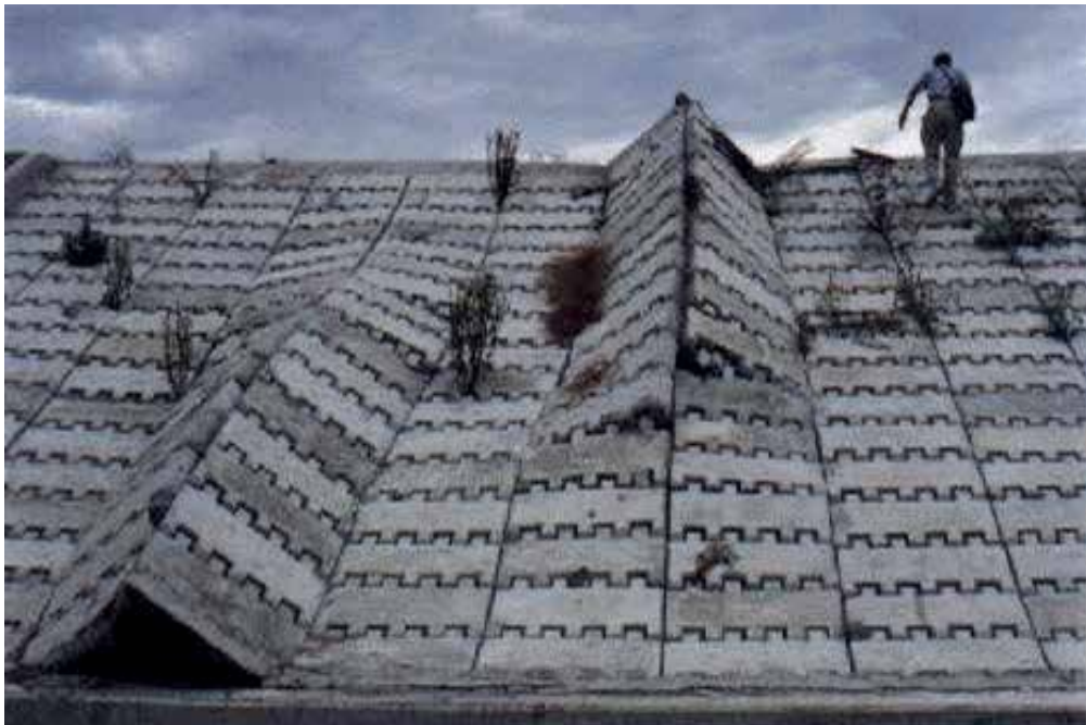
Figure 1. Buckling of river embankment lining after the 1999 Chi-Chi earthquake [32]
