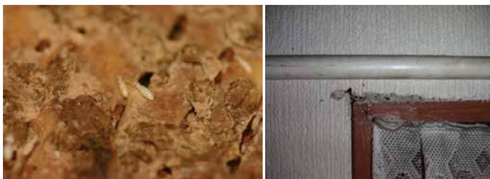
Fig. 1. Left: workers and soldiers of Coptotermes formosanus in their nest. Right: Damage on a residential structure caused by foraging termites of C. formosanus
