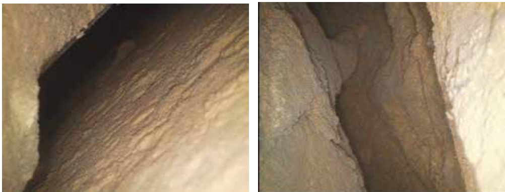
Fig. 16. Visualization of delamination in wall paintings by EverestVIT VideoProbe
