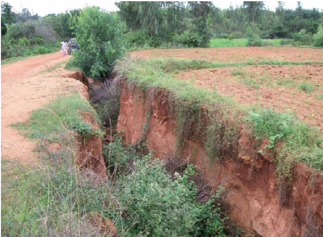
Fig. 10. Neglected road side water drain forming into a huge gully
