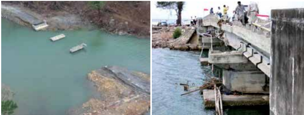
(a) Total Wash-Away of Deck (Unjoh, 2005) (b) Excessive Deck Displacement (Yim, 2005)
