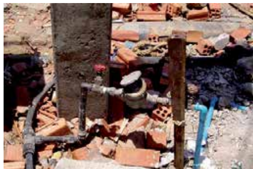
Photo 2. Water meter above ground. Black-colored polyethylene pipe is the service pipe of PWWA, and the blue-colored vinyl pipe is the residential pipe (Khao Lak, Thailand)
