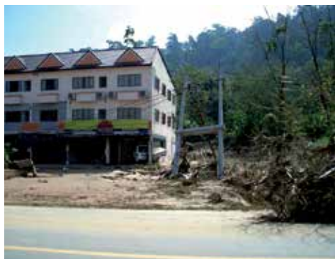
Photo 4. Electric pole tilted as a result of the scouring of the ground by the tsunami (Khao Lak, Thailand)
