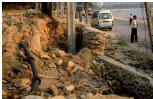
Photo 1. Exposed pipeline after scouring of embankment soil (Phuket, Thailand)
