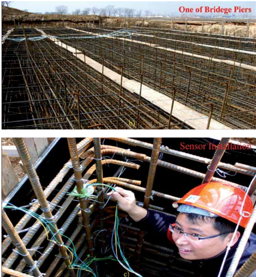
Fig. 32. Corrosion monitoring of the bridge pier. Scheme of the sensors' location a), Bird's eye view of the pier b) , and the sensor installation c)
