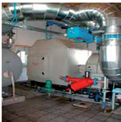
Fig. 1. Photograph of Altheim geothermal binary power plant in Austria (Ruggiero Bertani, 2007).
