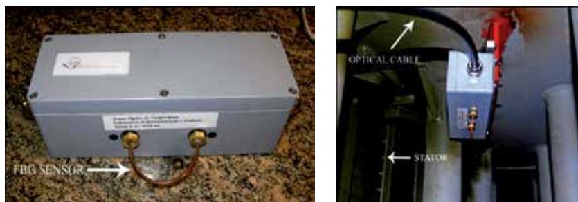
Fig. 3.5.4. Box containing the fiber-optic splices with the FBG inside the U-shape copper tubing (left) and installed inside the generator (right).
