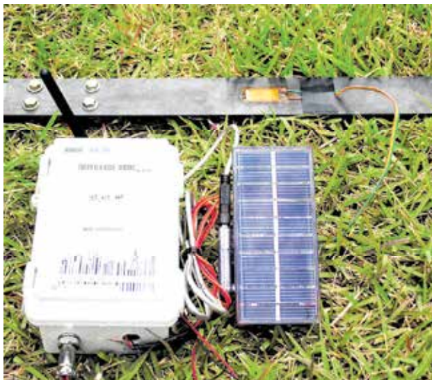
Fig. 6. Sensor node with a solar panel
