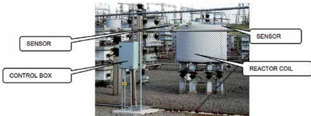
Fig. 3.1.7. The reactor coil and the sensors installed.
