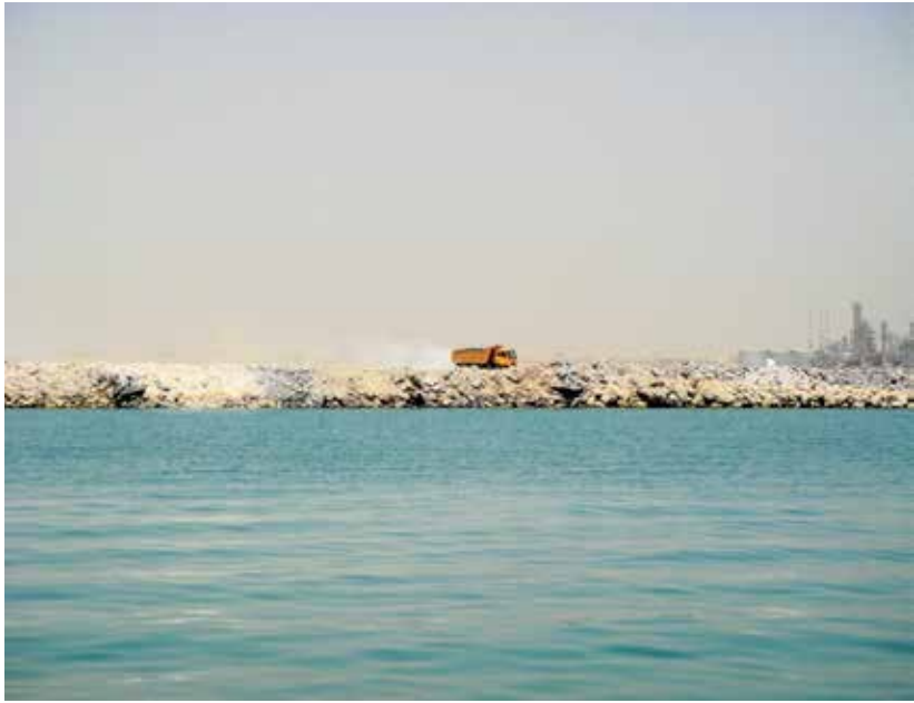
Figure 3. Rocks and sands extracted from nearby quarries are used to reclaim a coastal area along the eastern coastline of Bahrain (2012).
