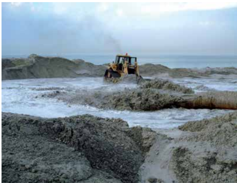
Figure 2. Sand and mud materials are pumped from a marine burrow area into the reclamation site. 'Dyar Al Muharaq' development in Bahrain (2013).
