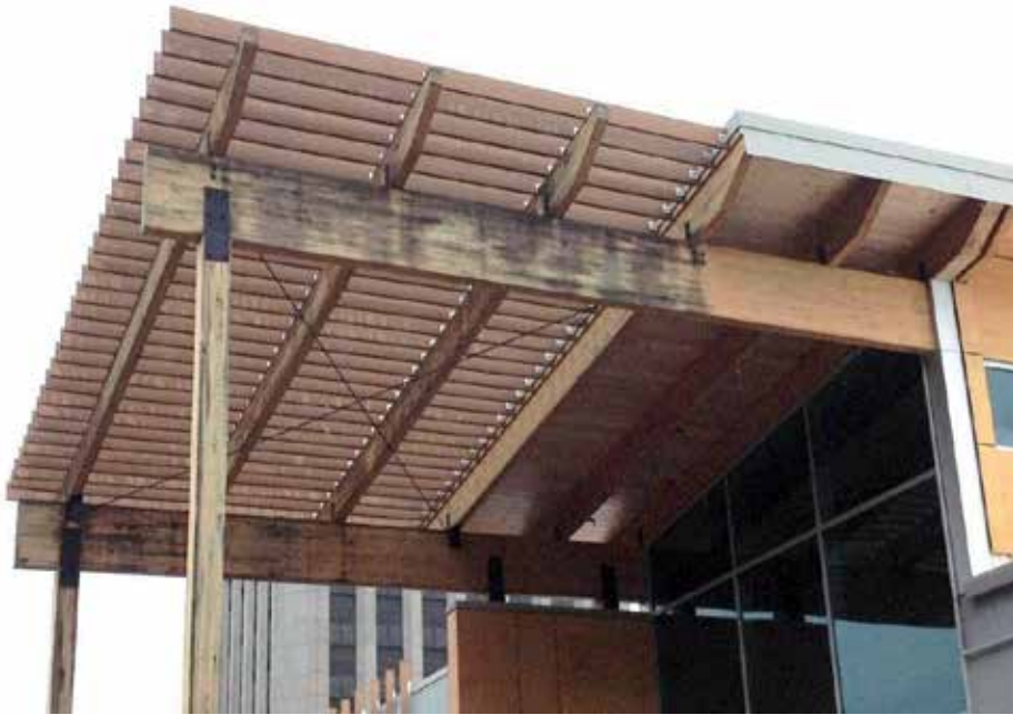
Figure 10. Illustration of the importance of roof overhangs for protecting wood from biodeterioration and corrosion. The right side of the beam is protected by the large roof overhang, whereas the left side is exposed to rain. SCALE: The beam supporting the trellis is 0.66 m deep.
