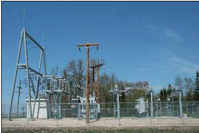
Fig. 1. Real electrical substation
