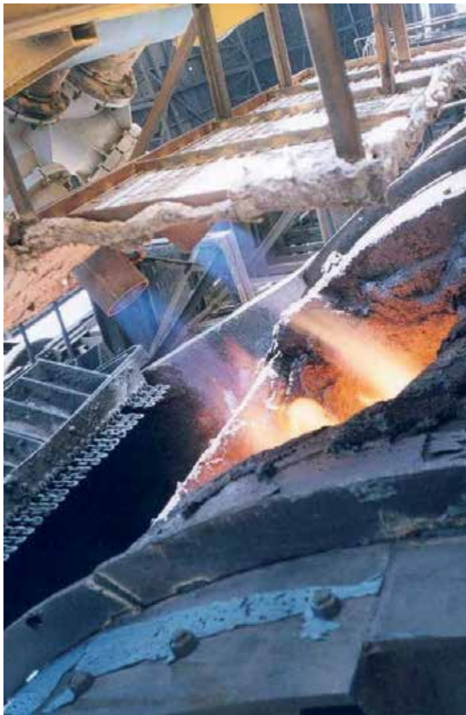
Fig. 7.1 Photo of Burners Installed in P&S Furnace
