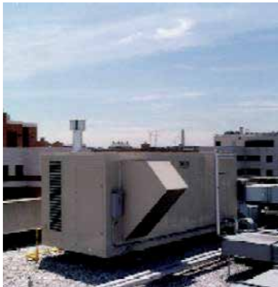
Fig. 8. A Desiccant Unit Atop the Park Hyatt Hotel, Washington D.C. (Source: National Renewable Energy Laboratory, DOE)
