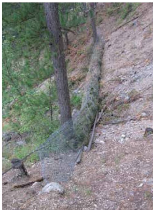
Figure 36. Example of use of a Fasnet eco-engineering work in the case study Val Drôme
