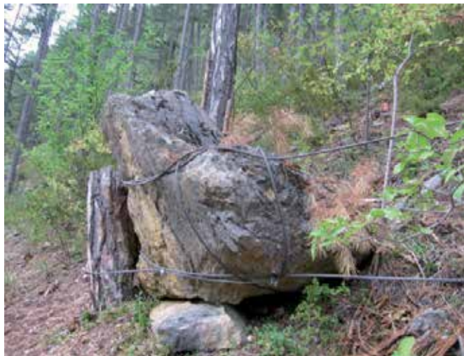
Figure 38. Example of anchorage of an unstable deposit rock in the Val Drôme case study.
