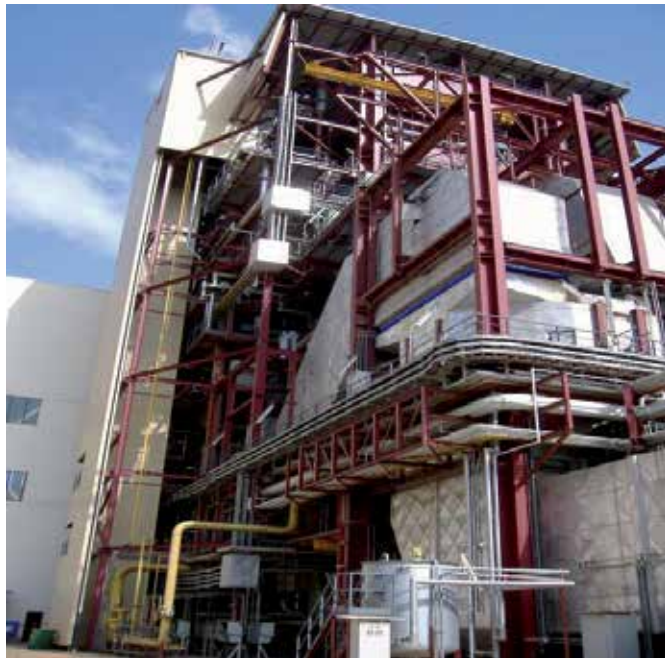
Figure 3. Example of a boiler of a TPP.
