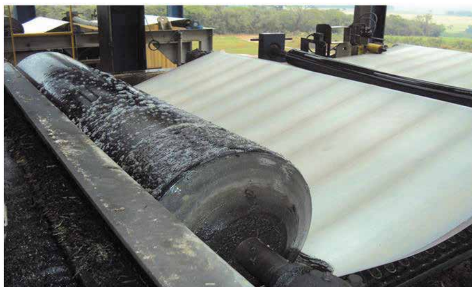
Fig. 5. Blanket type filter system (with suction strainer) to remove water and reduce moisture from the ashes
