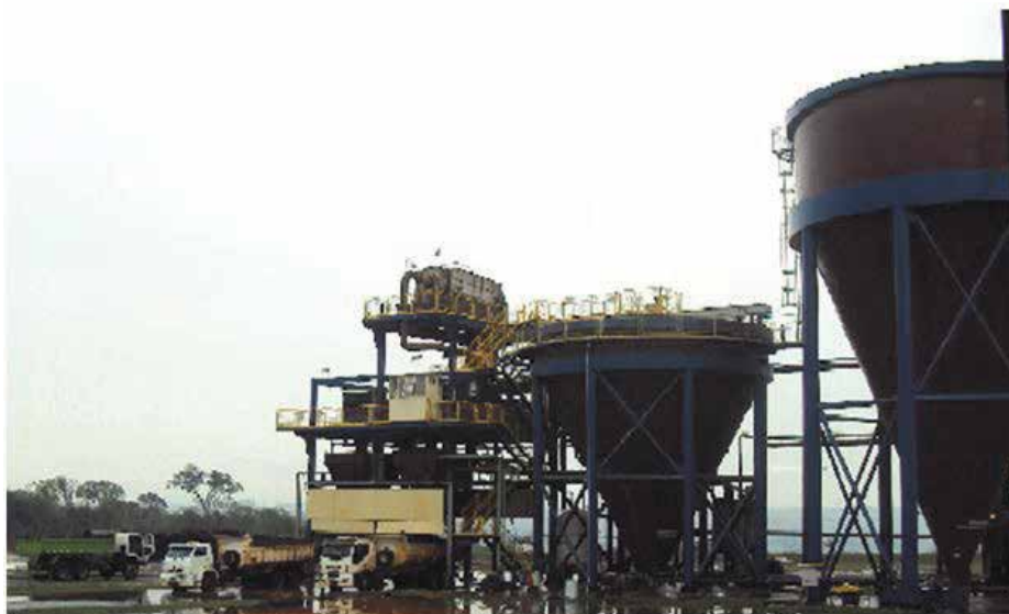
Fig. 4. System for treatment of water from gas washer to remove the ash using decanters and porous blankets.
