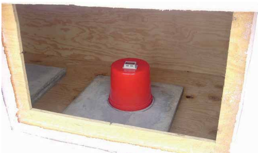
Figure 3. Mini-roof system showing temperature sensor installed inside a mini-roof.
