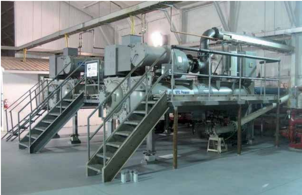
Figure 1. Photograph of Chena ORC-based geothermal power plant at Chena, Alaska, USA (Holdmann, 2007).
