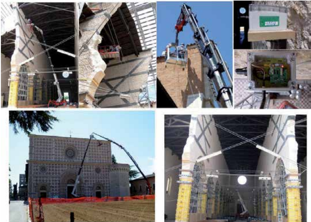
Figure 12. Installation phases of the monitoring system at the Basilica di S. Maria di Collemaggio: a) b) sensor positioning on the central walls of the nave, c) sensor positioning beyond the facade, d) f) sensor views, g) phase of on-site testing, h) sensor positioning at the end of the nave walls.
