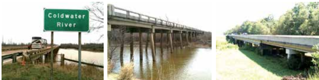
Figure 5. Three bridges crossing the Coldwater River on lifelines serving the study area; (left) view of southbound I 55 bridge; (middle) nearby US 51 bridge showing piled bents carrying simple spans; (right) view of northbound US 78 bridge
