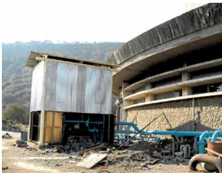
Fig. 4. Desalination unit located outside Cirus annulus area
