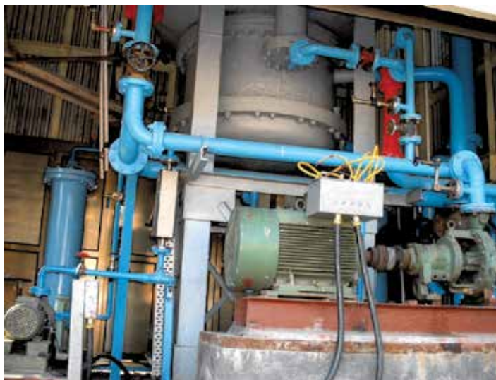
Fig. 3. Evaporator section of Desalination unit and Booster pump
