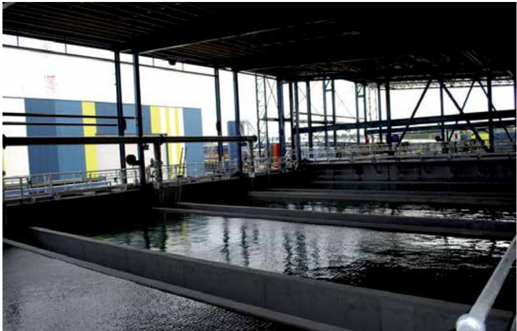
Fig. 25. Gravity dual media filters (Australian desalination plant)
