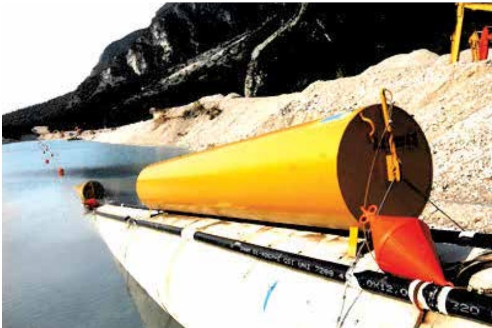
Fig. 2. Launch of a submerged methan pipe. The buoys along the launched length are in full view.
