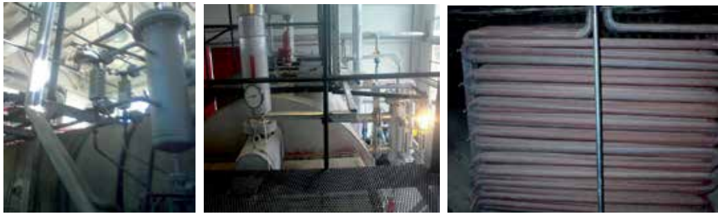
Fig. 3. Superheater of the heat recovery steam generator at 2xST 18 Cogenerative Power Plant
