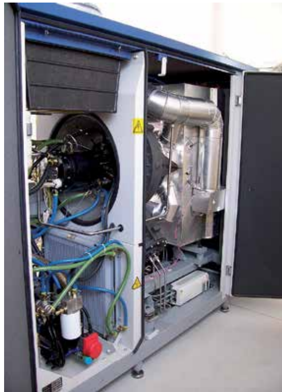
Fig. 2. The T100 power module installed at the laboratory of the University of Genoa (power electronics and control system are not shown).
