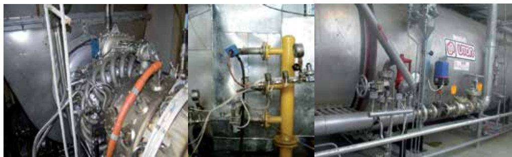
Fig. 2. ST 18 gas turbine (left), afterburning installation burner (centre) and heat recovery steam generator (right) at 2xST 18 Cogenerative Power Plant
