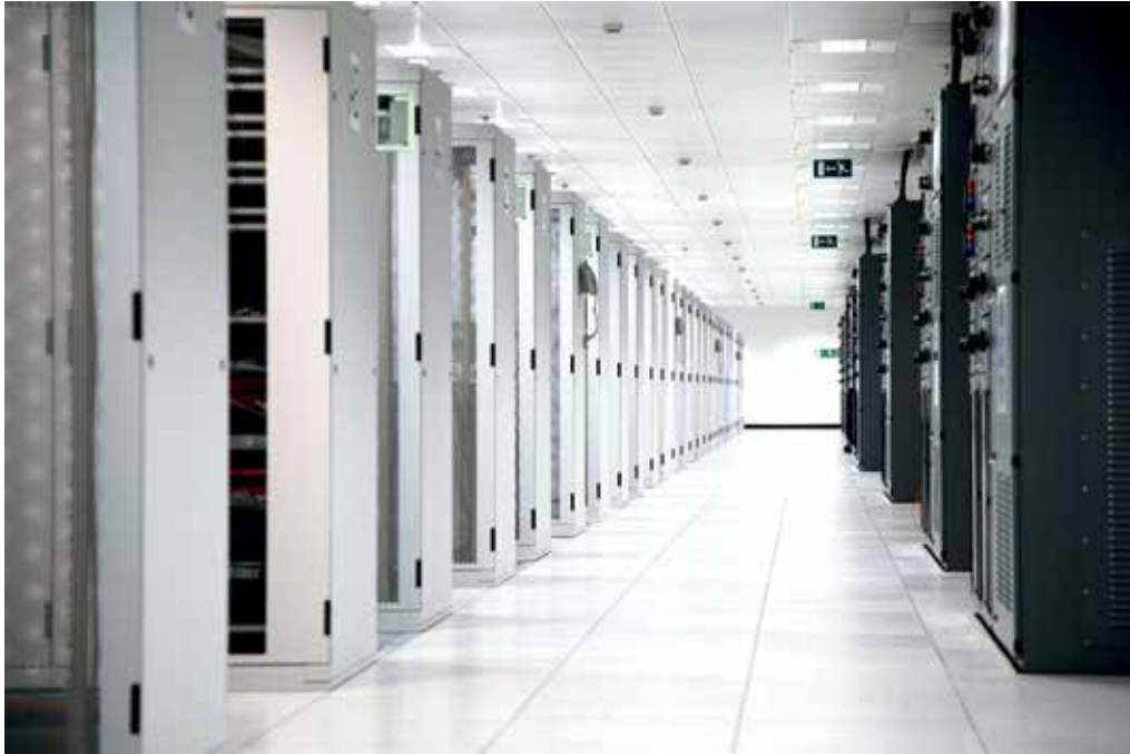
Fig. 1. A large scale data centre with several rows of server racks
