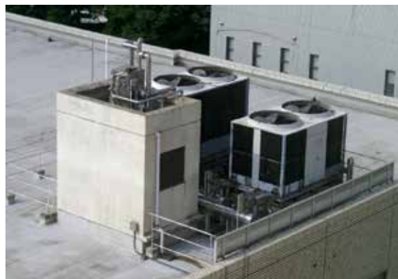
Fig. 14. Heat pump - chiller units
