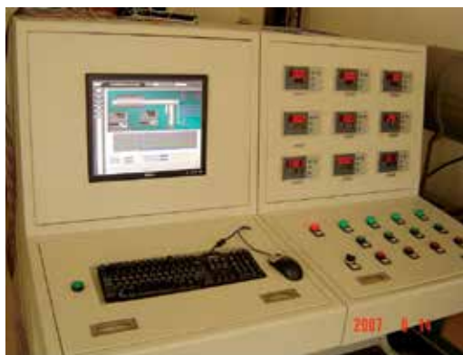
Fig. 12. Monitor equipment of heat pipe technology
