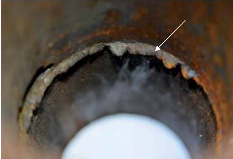
Figure 14. The inner side of circle area in Fig. 11 showing an excessive overfill (arrow) in the failed pipe at 12 o'clock position.
