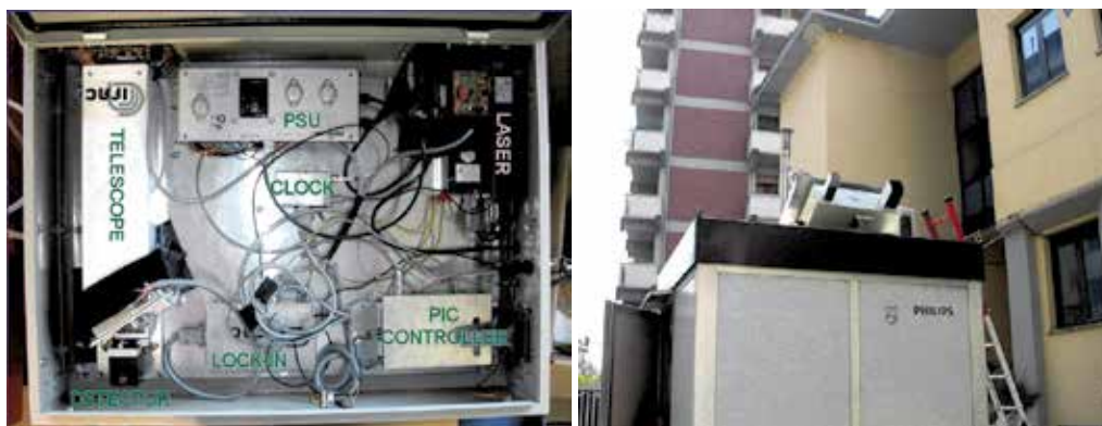
Fig. 12. The instrument opened (left) and installed on the roof of the ARPAT, PM-monitoring station in Florence (I) (right)
