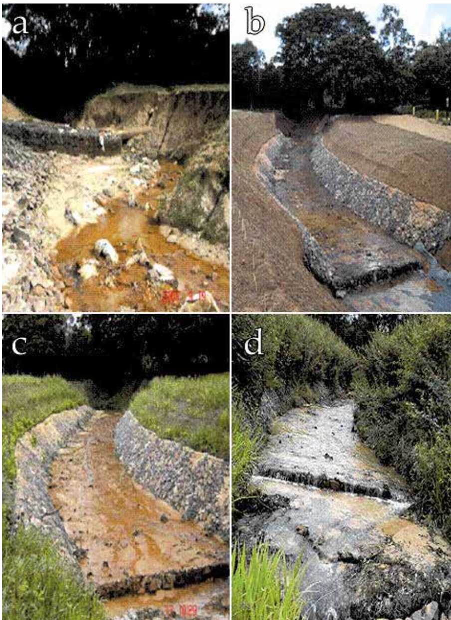
Fig. 4. Stages of installation of the biotechniques in Paramopama Creek in northeastern Brazil. a) Degraded river channel and riparian zone; b) Gabion at the toe and at the river bed, plus jute matting at the streambank; c) Development of the grass cover; d) Vegetation development six months after installation, composed by legume-shrubs mixture. Adapted from Holanda et al., (2009).
