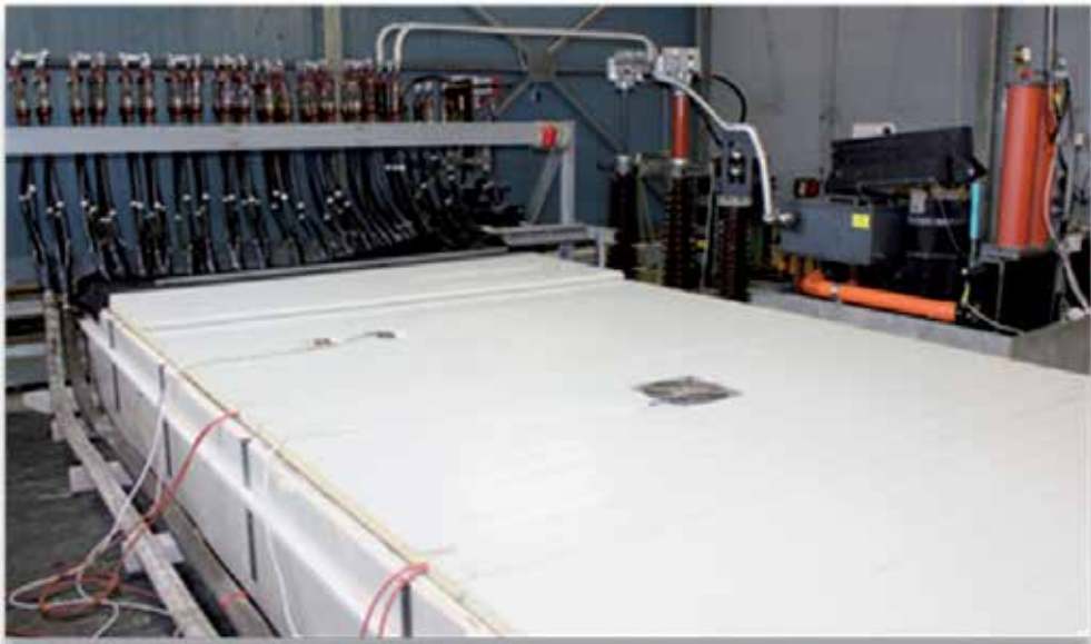
Figure 11. Partial overview over central components of the ICAAS system (transformers for voltage and current generation, overvoltage protection, rectifiers, etc.) and cable samples
