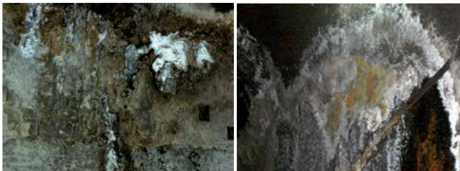
Fig. 1. Deterioration of railway tunnel (Southwestern Region, China)
