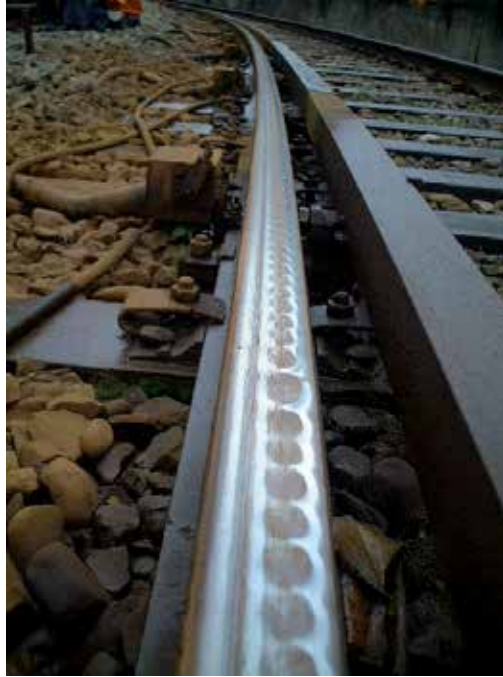
Fig. 2. Example of rail corrugation
