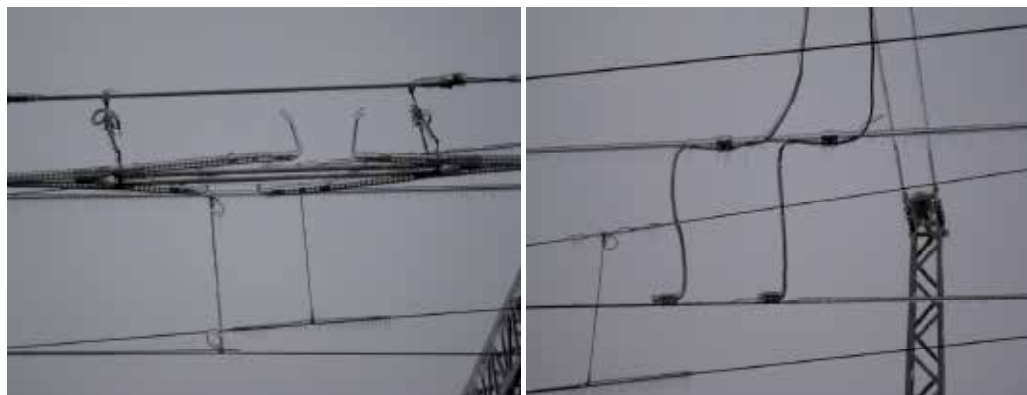
Fig. 1-2. Icing of overhead contact wire
