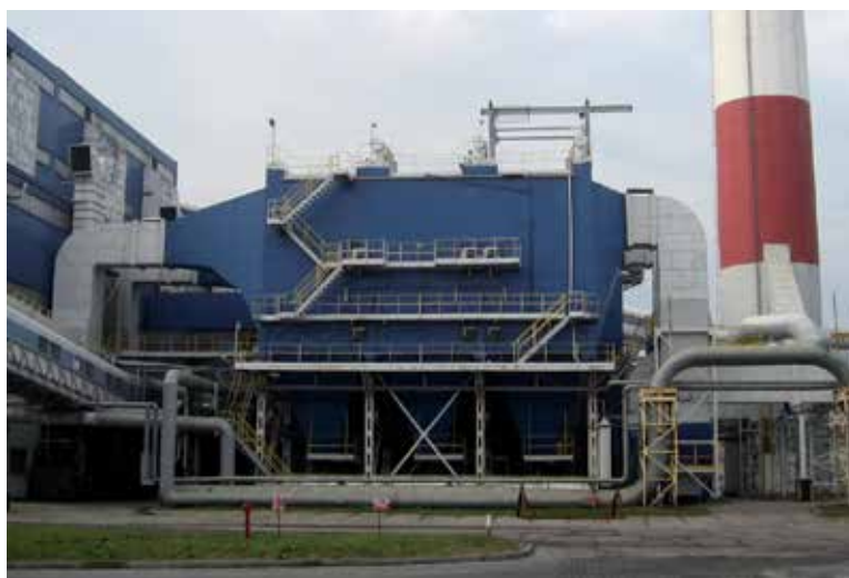
Fig. 1. Electrostatic precipitator in Thermal-Power Station.
