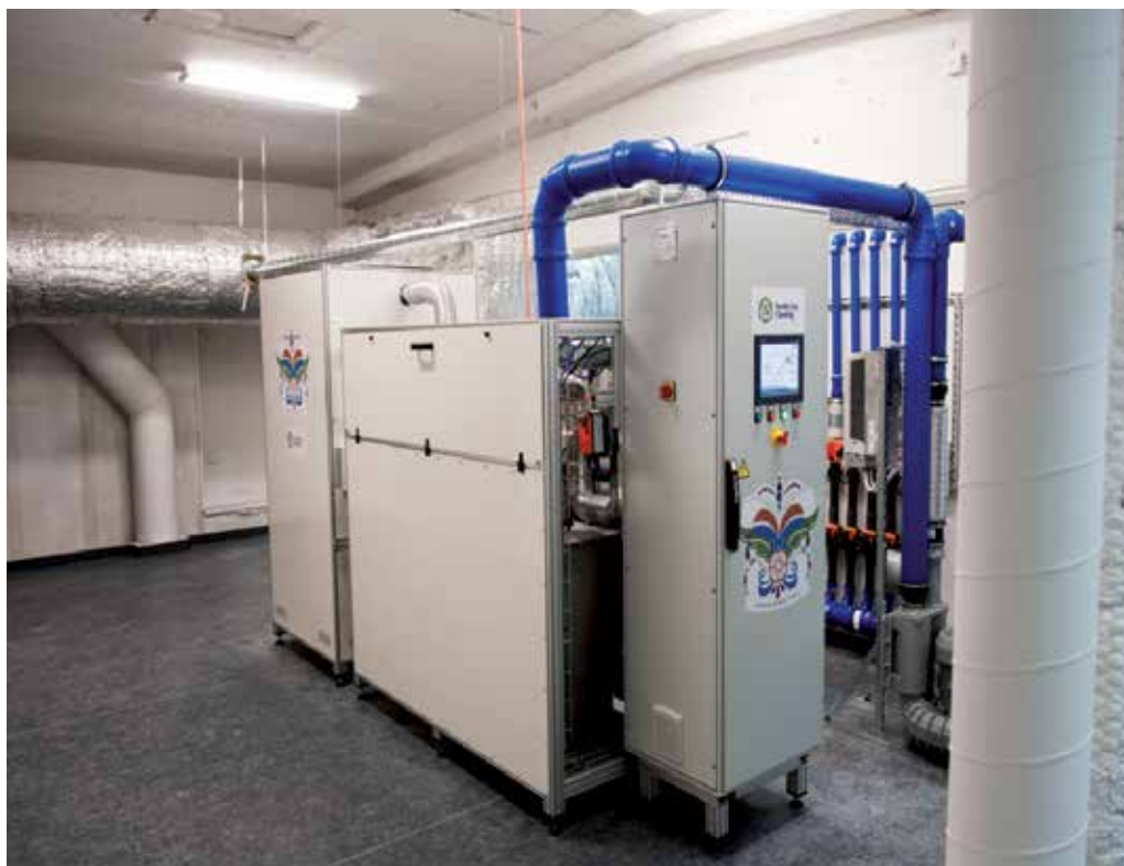
Fig. 4. The unit from NGC installed at Södertälje hospital. (Photo Anette Andersson)
