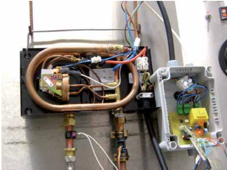
Fig. 3. Photo of the electric water heater and the micro-controller board.
