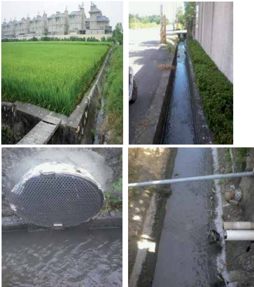
Picture 5. Community sewage directly drains to irrigation waterways
