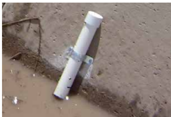
Fig. 7. Installed Hobo Pressure Transducer
