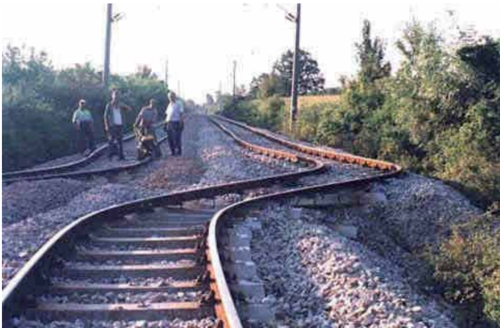
Fig. 9. An example of rail way which build on fault zone and is cutted by this zone in Turkey after 1999 Marmara Earthquake. It is taken from http://www.resimkarikatur.com/resim1684.html . Photographer is unknown.
