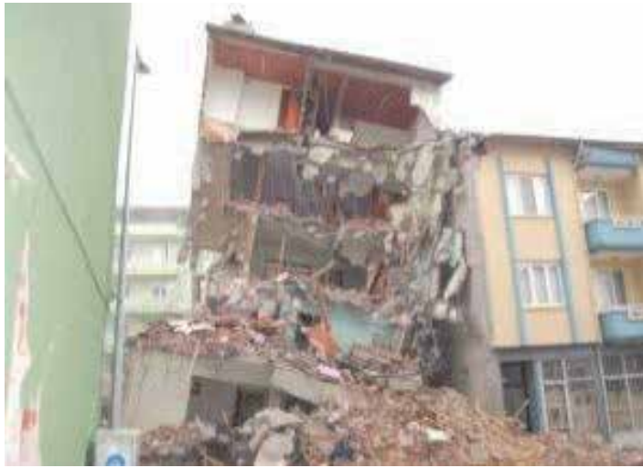
Fig. 10. An example of collapsed structure because of building design and different construction height after 1999 Marmara Earthquake. It is taken from http://www.haberingundemi.com/haber/Depremin-Simgesi-Bina-Yikildi/80399 . Photographer is unknown.
