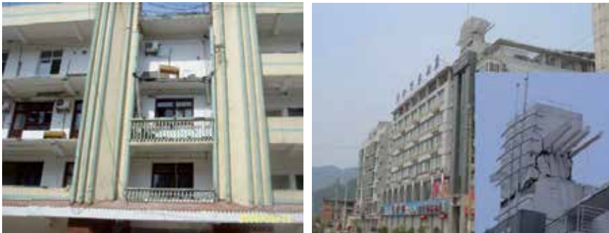
Fig. 5. Falling of the corridor fence and horizontal crack of the protruding member
