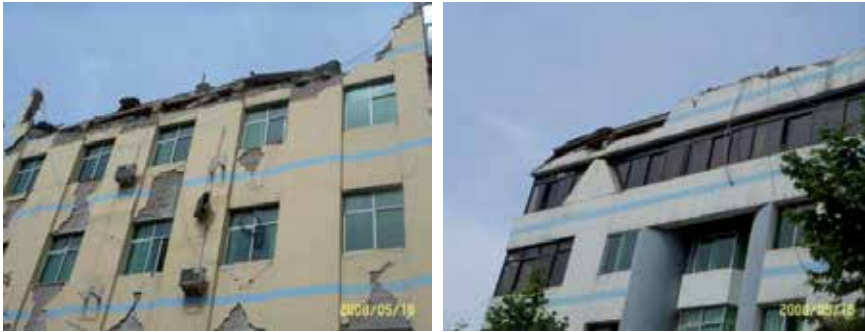
Fig. 4. Failure of the parapet wall
