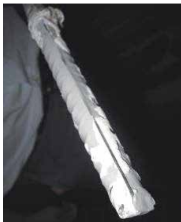
Fig. 19. Interlocking surface in an anchor installed into a hole which is not filled with epoxy (Photo by Dr. Halil Nohutcu)
