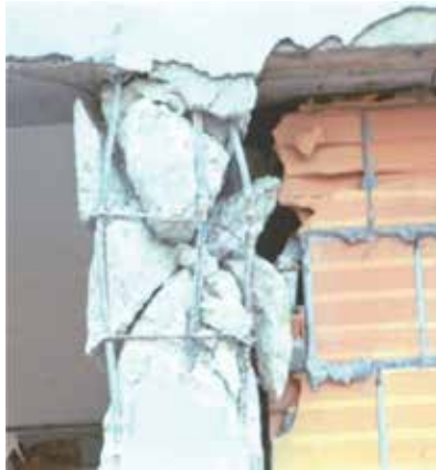
Fig. 9. Shear failure of column (Italia 2002)
