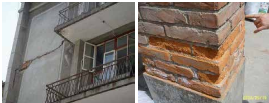
Fig. 2. Horizontal cracks on the wall or the bearing brick column
