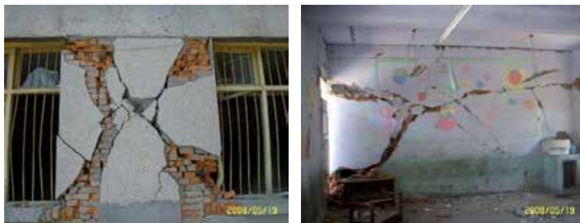
Fig. 8. Through cracks on the longitudinal and transverse load-bearing wall
