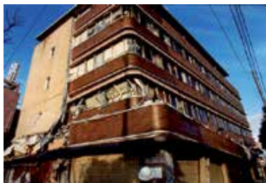
a) Torsional failure of structure (Kobe, 1995)
