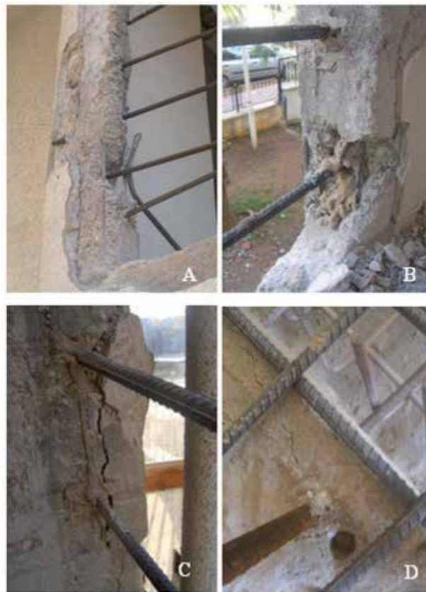
Fig. 18. Poorly implemented anchor examples (A, B: anchors implemented on defective surfaces; C: Anchor implemented near a crack; D: Anchor fracturing the concrete during the tensile test)
