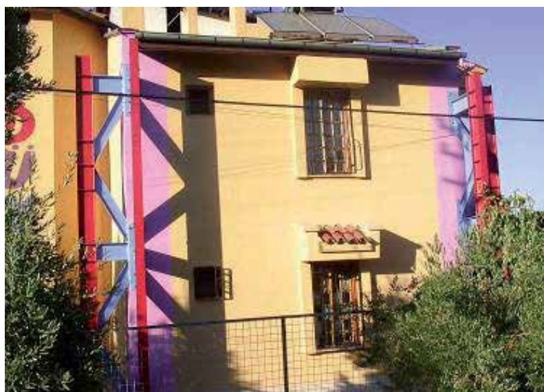
Fig. 11. Buttress type external steel shear wall (Photo by Dr. Yavuz Selim Tama)
