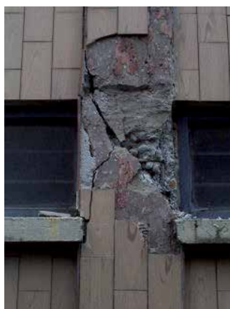
Fig. 8. shear failures in columns (California 1994)
