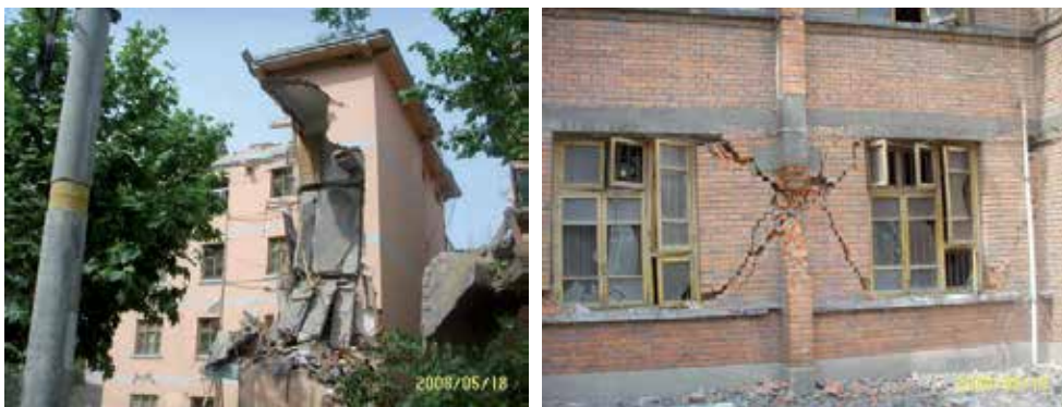
Fig. 1. Through diagonal or X-shape cracks on the wall
