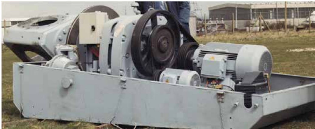
Fig. 16. Drivetrain of the Windharvester wind turbine.
