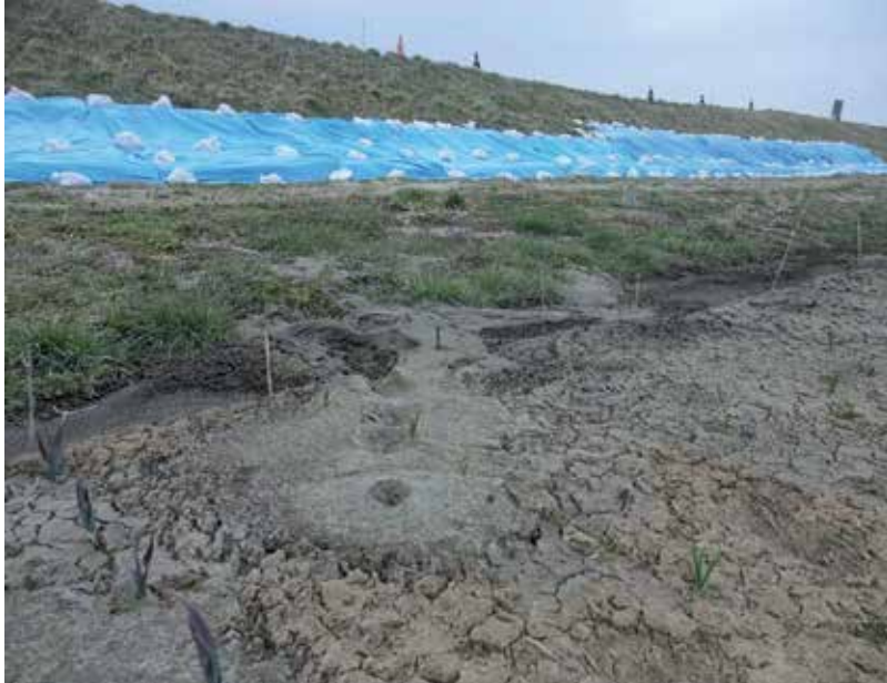
Fig. 44. Levee Slope Repair and Sand Boils at Toe, Japan. (JSCE 2011)
