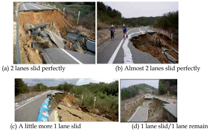
Photo 3. Large-scaled damage of road embankment without traffic performance
