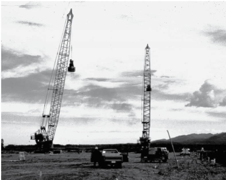
Fig. 6. Deep Dynamic Compaction to prepare a gravelly sand foundation soil for the reconstructed Jackson Lake Dam, Wyoming. Reprinted with permission from Handy and Spangler (2007), The McGraw-Hill Companies, New York.
