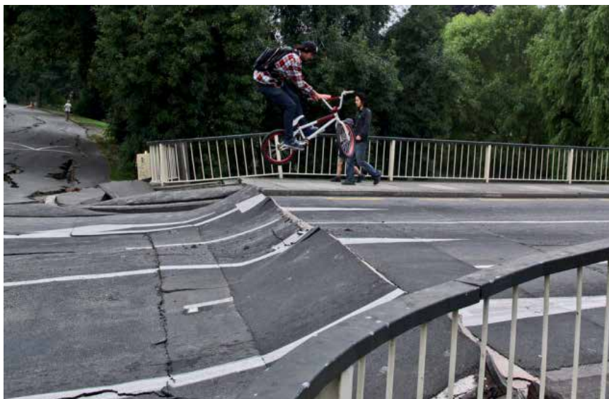
Fig. 47. Settlement of Approach Fill at Bridge Abutment Formed a Bike-Jump for a Youngster. http://otilya.com/view/News/Asia-Pacific/New-Zealand
