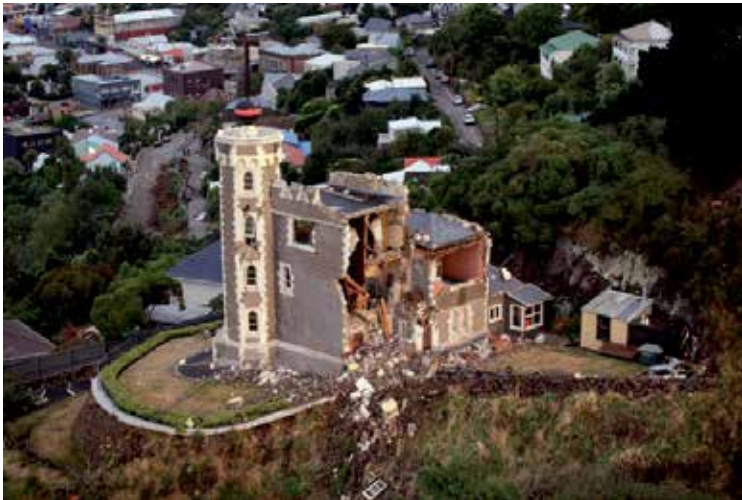
Fig. 30. Topographic Amplification May Play a Role in Damaging an Unreinforced Masonry Building, 2011. http://otilya.com/view/NewsAsia-Pacific/New-Zealand
