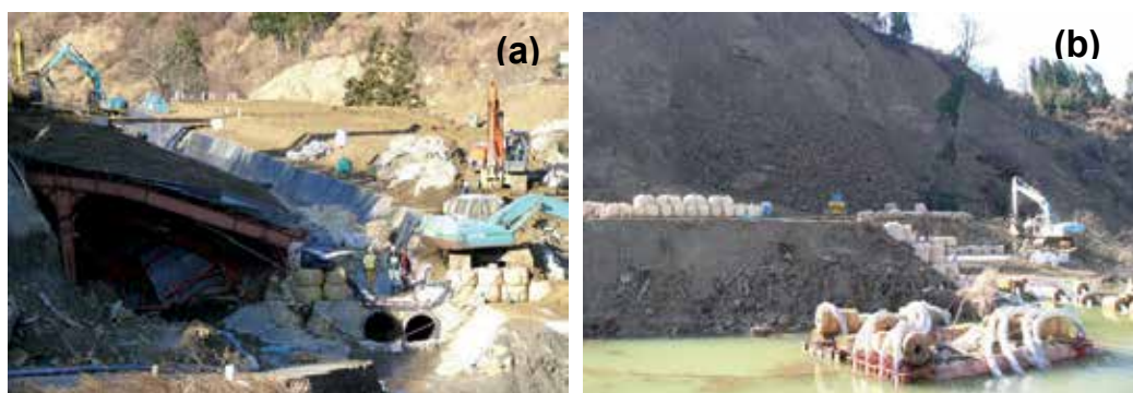
Fig. 4. Emergency works at Higashi Takezawa landslide dam. Photo taken on 20.12.2004 by Takeji & Tadashi, 2005
