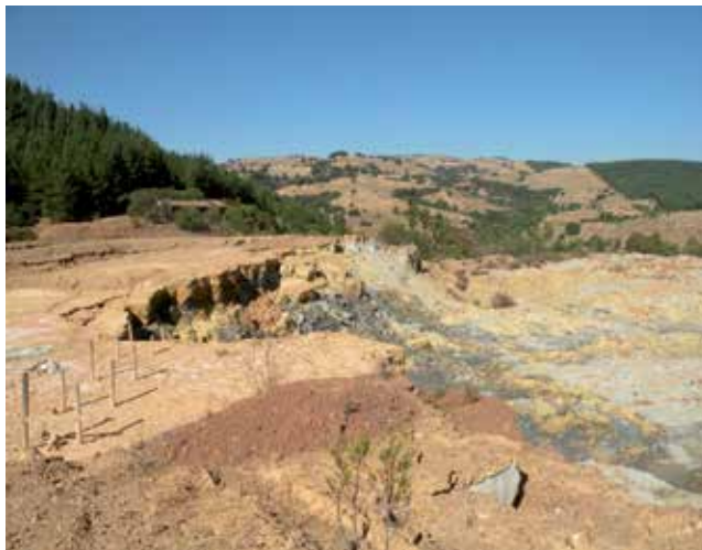
Fig. 24. Upper Scarp of Failed Tailings Impoundment. (GEER 2010)
