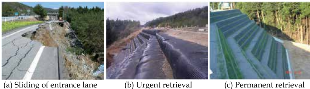
Photo 4. Damage and seismic retrieval with geotextile
