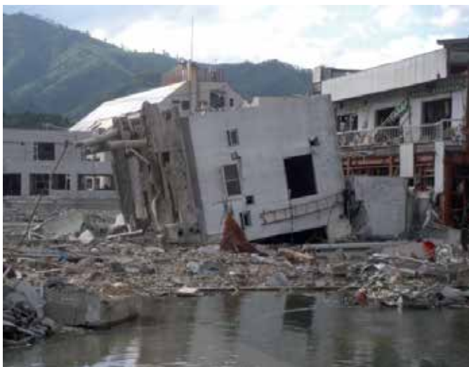
Fig. 38. Overturned Police Station, Onagawa, Japan, 2011.
