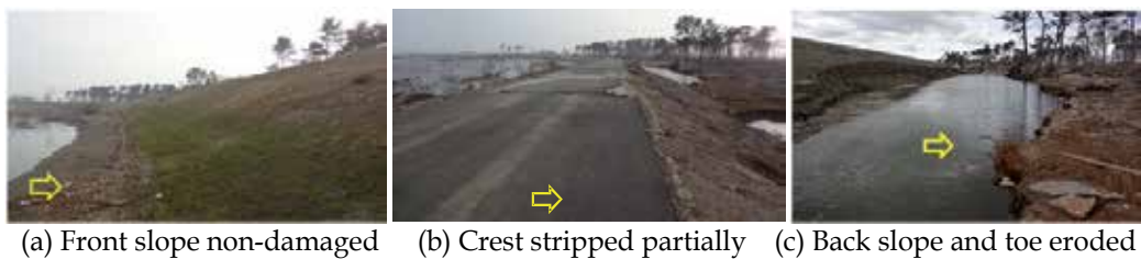
Photo 8. Dyke overflowed by tsunami
