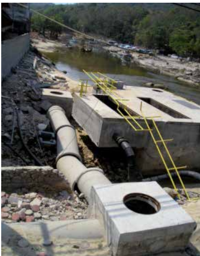
Fig. 39. Pump Station Damaged by Wave Scour, Patong Beach, Phuket Province, Thailand, 2004.
