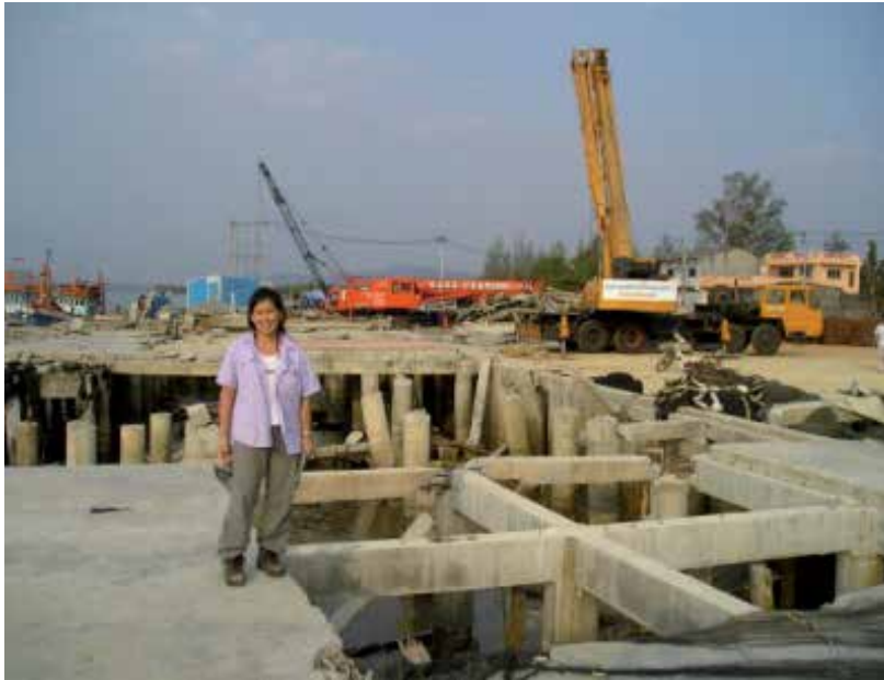
Fig. 36. Wharf Damaged by Wave Impact and Uplift, Bam Nam Kem, Phang Nga Province, Thailand, 2004.
