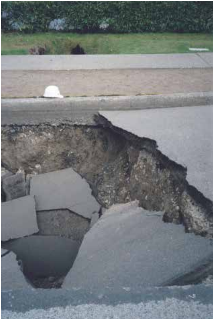
Fig. 46. Sinkhole Formed by Collapse of Roadway During Earthquake, Washington, 2001.
