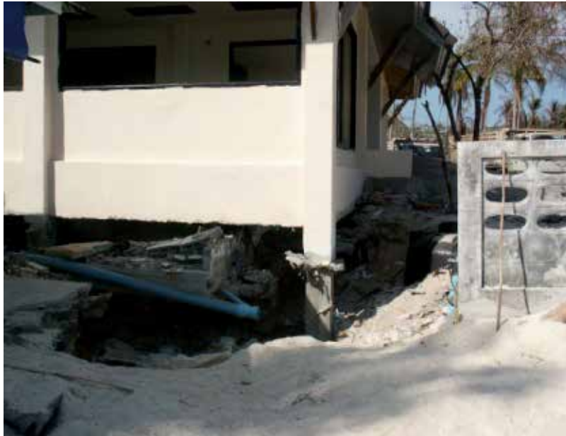
Fig. 40. Scouring of Foundation Soils and Severing of Building's Utility Lines, Phi Phi Island Hospital, Thailand, 2004.
