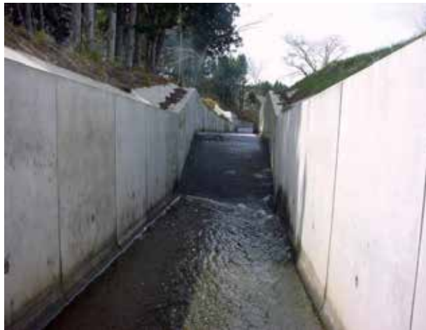
Photo 6. Drop work is constructed for moderation of channel slope, opposing swimming up of fishes
