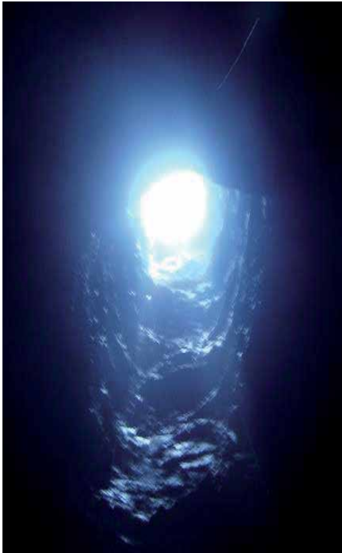
Fig. 4. Profile of pilot surge shaft excavated by long hole raise driving at Koilsagar
