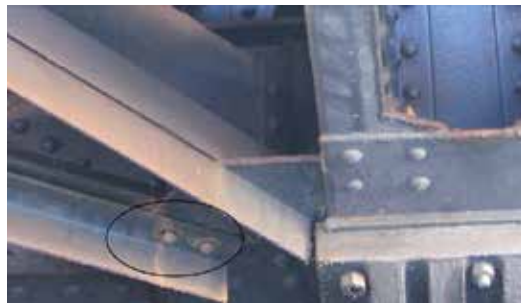
Fig. 7. Inefficient joints – railway bridge on a main line
