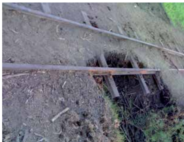
Fig. 17. Soil Erosion under the railroad.
