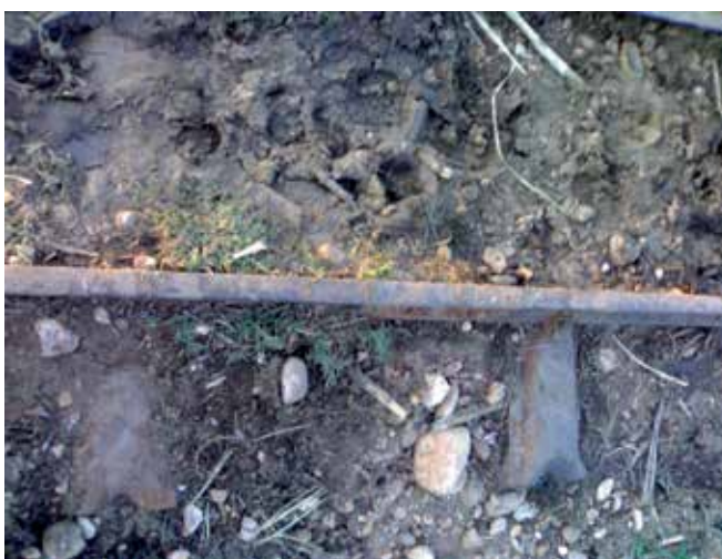
Fig. 16. Balastless narrow rail track showing intensive ruste of sleepers buried in the clay soil
