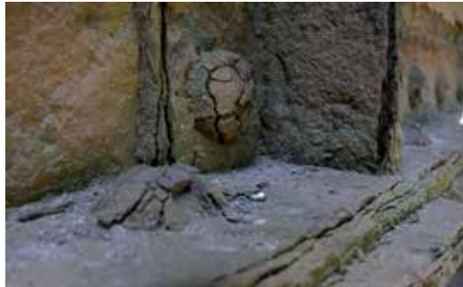
Fig. 6. Strong corrosion at the lower flange – railway bridge on a main line
