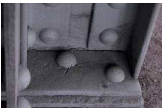
Fig. 4. Crack in the lower flange near to the bearing
