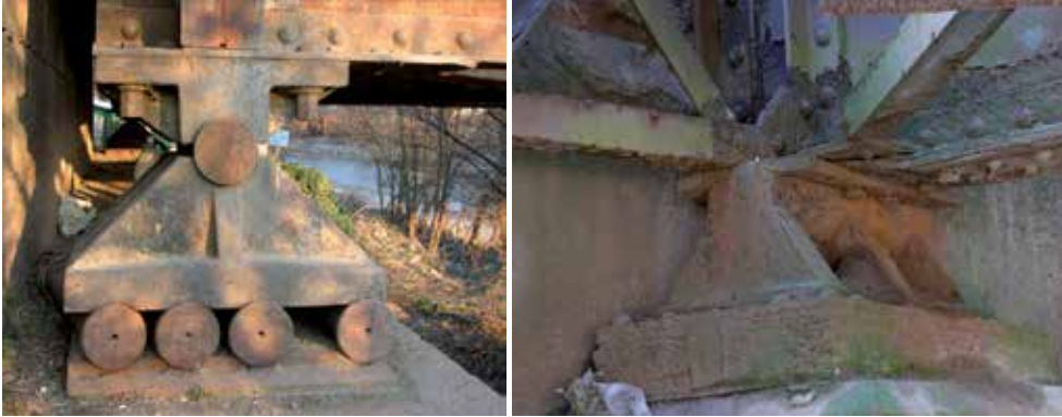
Fig. 5. Defects on bearings
