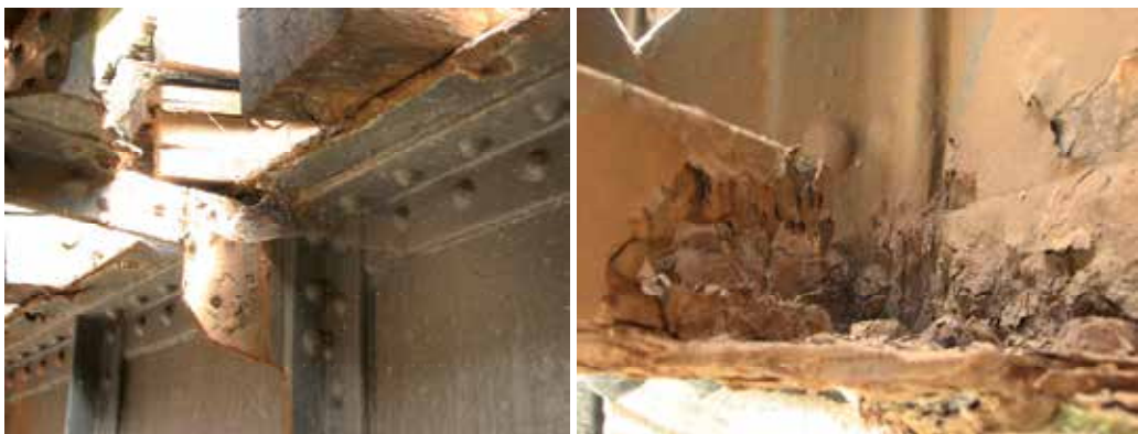
Fig. 34. Corrosion attack details
