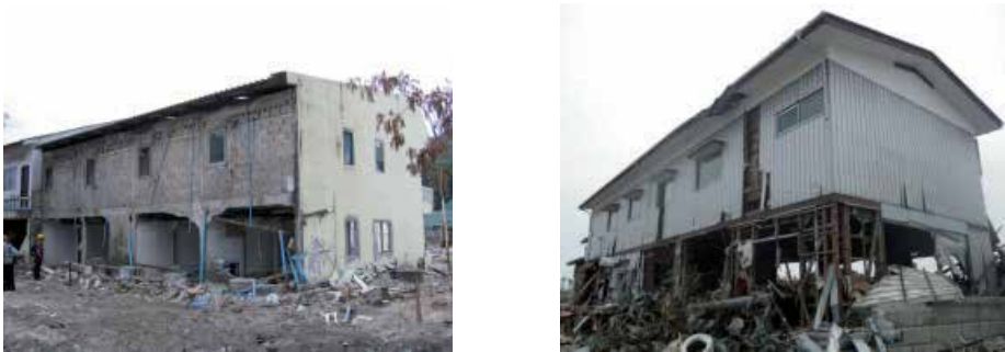
Fig. 25. Examples of building damage in the case of the 2004 Indian Ocean tsunami in Thailand and the 2011 Tohoku tsunami in Japan
