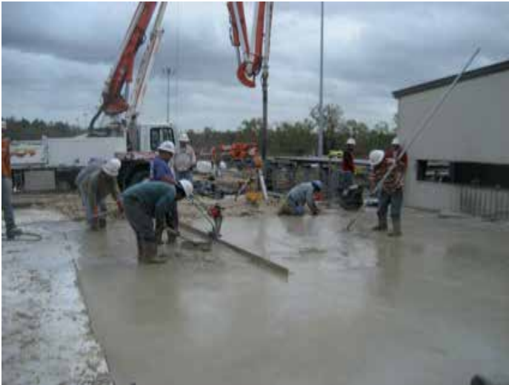
Fig. 4. Construction of base for a heat treating facility in Houston, Texas. Cycling of temperatures caused severe breakdown of conventional concrete, (James K. Hicks, et. al., 2009).
