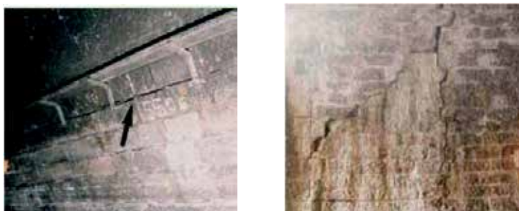
Fig. 9. Illustration and examples of degradations of masonry tunnels.
