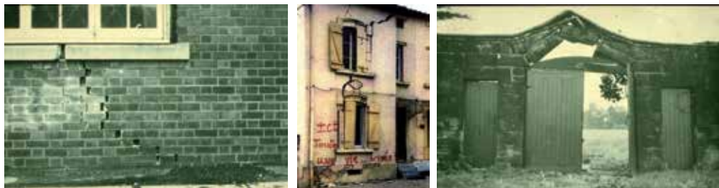
Fig. 18. Damages induced by compression strain due to soil subsidence (Deck et al., 2003).
