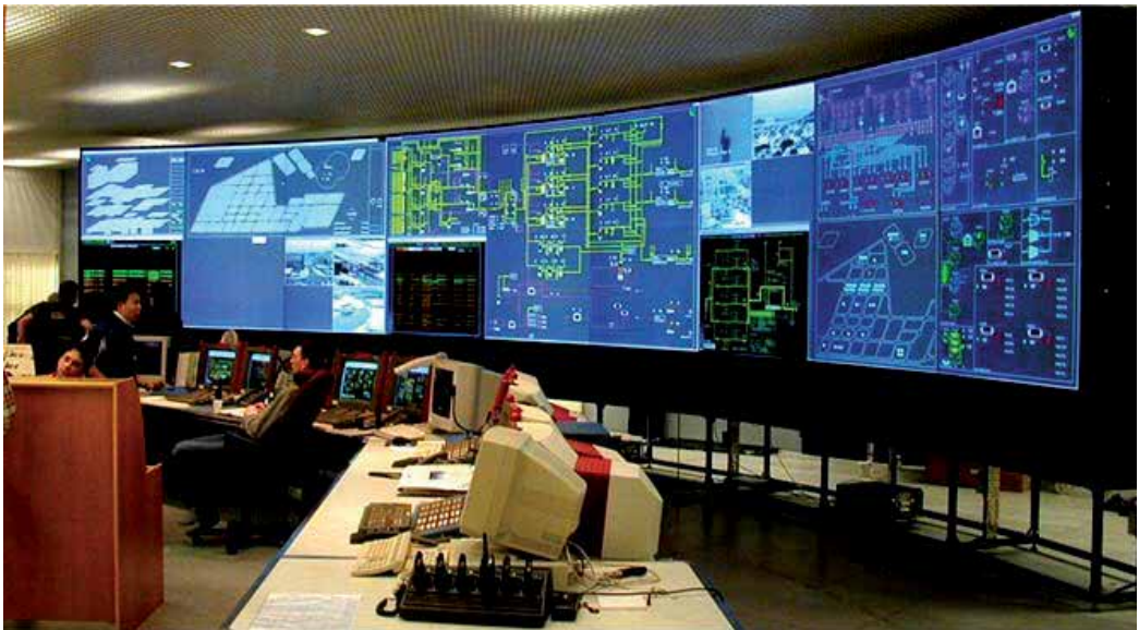
Fig. 4. Large display walls make it possible to present a plant overview for the operators.
