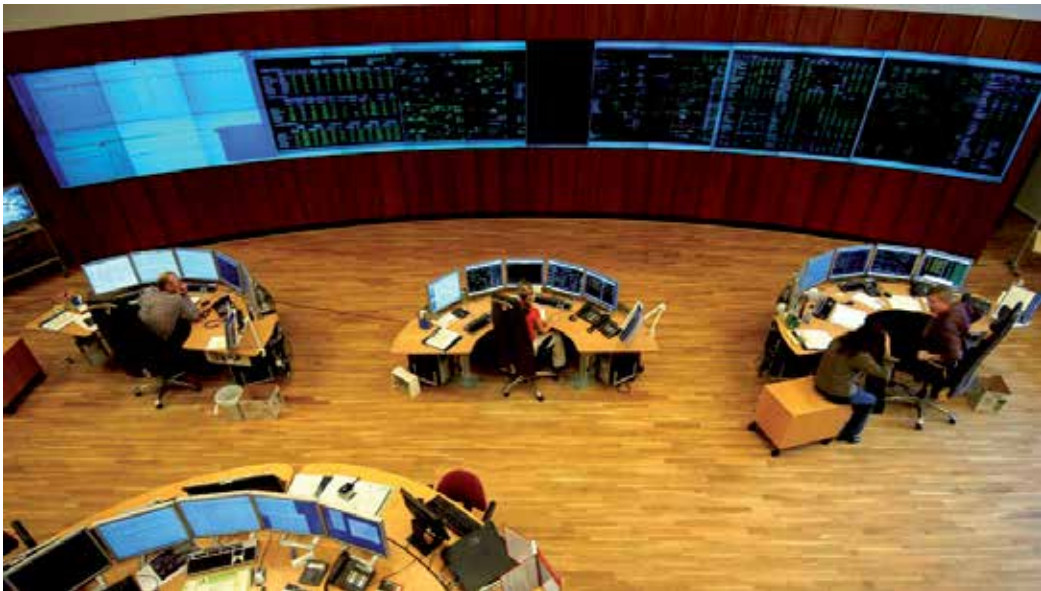
Fig. 7. Large display walls have a great impact on the control room layout.
