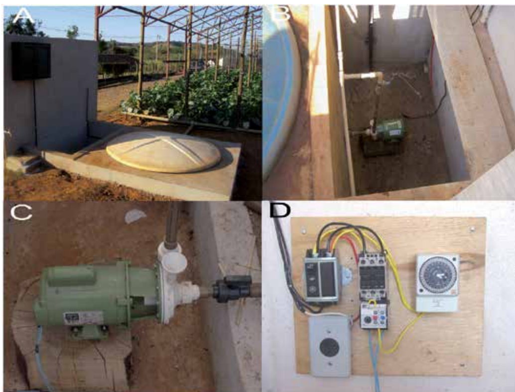
Fig. 2. Detail of the pump house (under construction) illustrating: A) Hydroponics being built by focusing the detail of water tank buried in the soil to avoid heating, B) and C) Set motor pump installed in a primed (below the level of reservoir), D) Panel containing outlet, timer relay and nutritious species. Photos: IFMG Bambuí, Professor Ricardo M. Corrêa.
