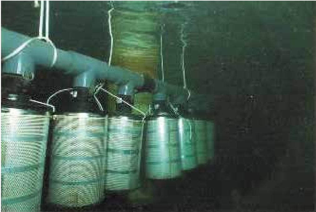
Fig. 4. UCC vacuuming filtration system underwater manifold.
