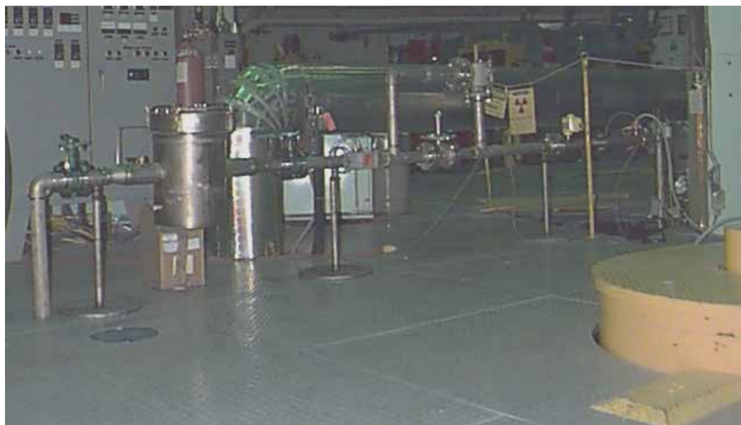
Fig. 8. Vent line for EBR-II Primary Tank with installed instrumentation and HEPA filter.
