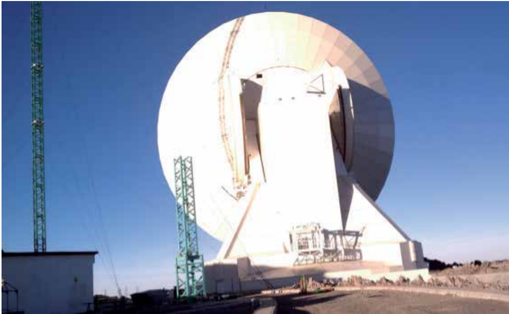
Fig. 6b. The GMT ( http://www.lmtgm.org/images/sitepics05012011/LMTatSunrise1.jpg ) observatory construction site, with the last ring of the antenna in the process of installation.
