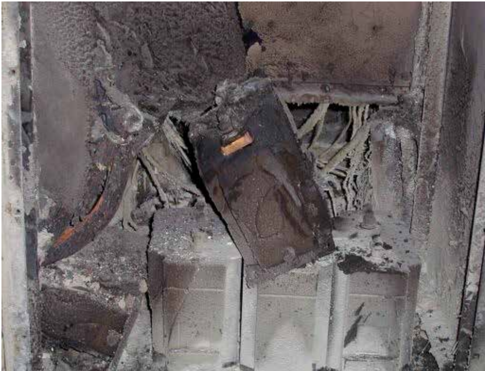
Fig. 4.3.1. Damage to the PT and panel where PT was connected.
