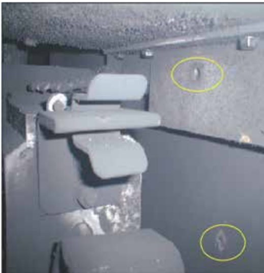
Fig. 3.5.2.2. Arc flash evidences between CT's and metallic walls.
