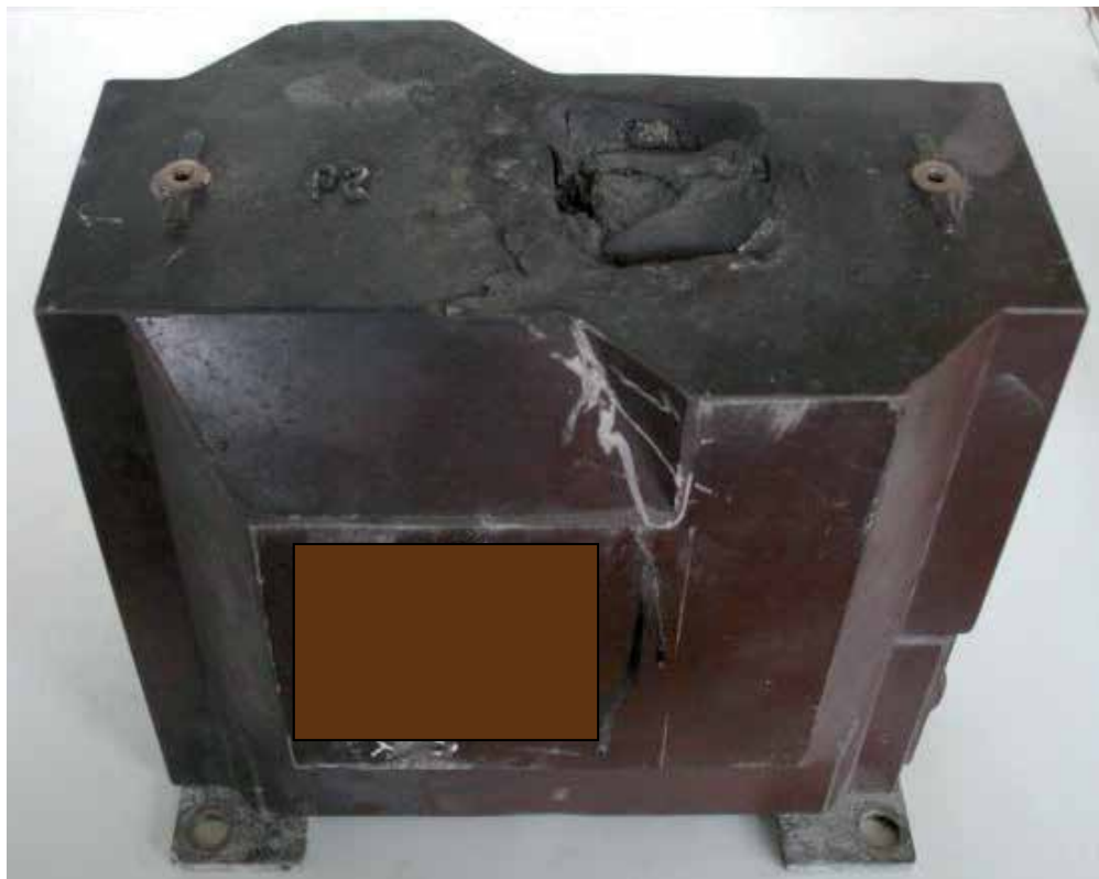
Fig. 4.3.2.1. Potential transformer that caused the failure in switchgear.
