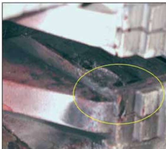
Fig. 3.5.1.2. Damages evidences in the stator core laminations of TG-2.
