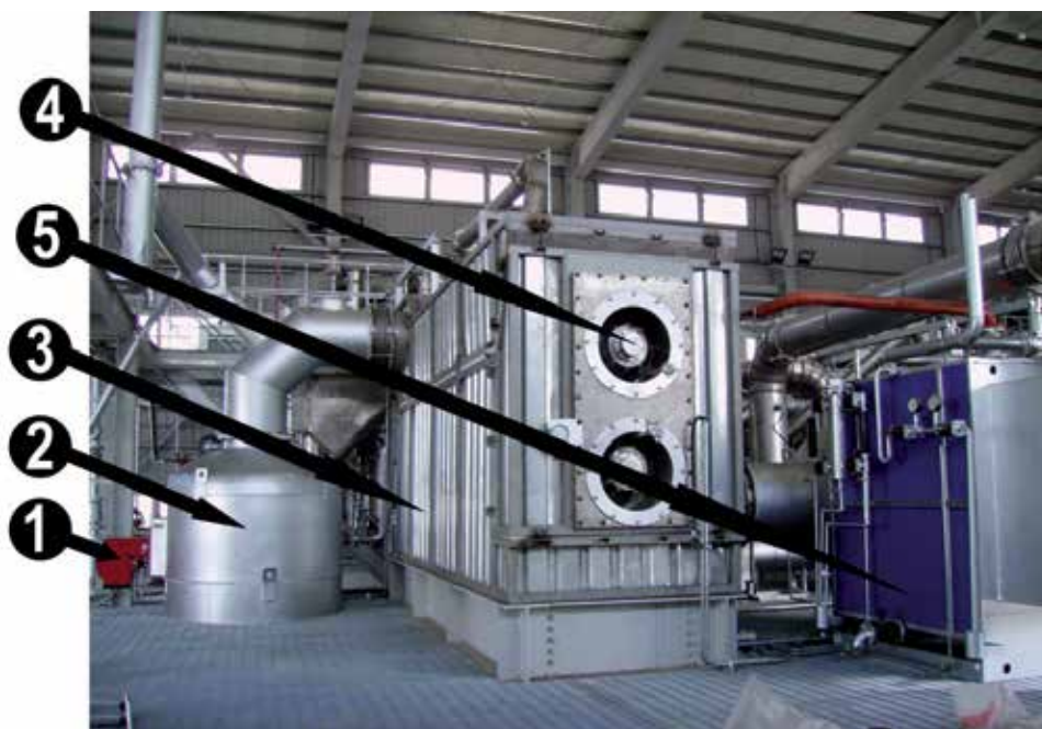
Pict. 1. ENRESTEC thermal units for waste tire pyrolysis with steam: 1 - oil fuel burner, 2 - furnace, 3 - pyrolysis reactor heating box, 4 - double-screw reactor in the box, 5 - second heat steam boiler.
