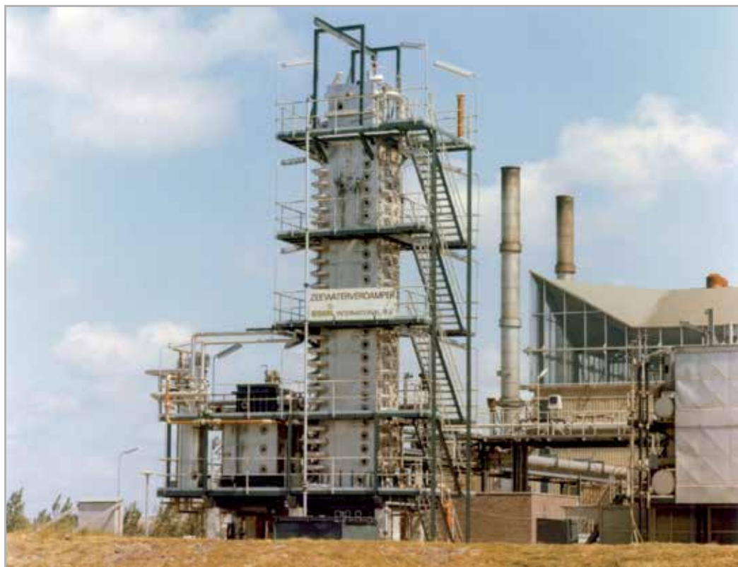
Fig. 11. MSF / FBE evaporator, Isle of Texel.
