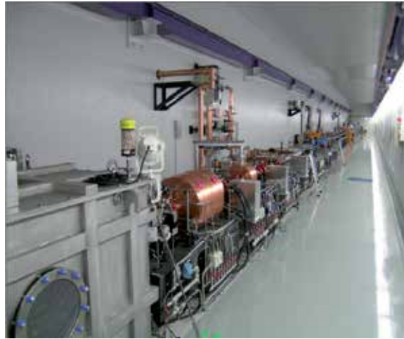
Photo 4.1. SCSS prototype FEL facility (view from the gun to the dump)
