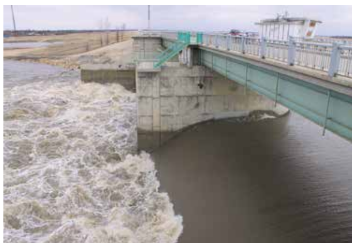
Fig. 8. The Winnipeg Floodway (Photo: Courtesy of Manitoba Floodway Authority, 2011)
