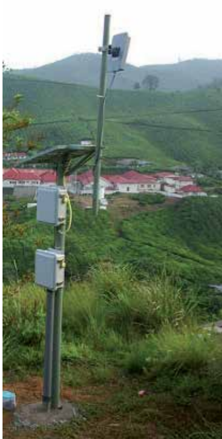
Fig. 8. C3 Sensor Column of Main Deployment
